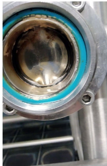
Figure 6 Flange on the pipe overgrown with active biofilm
