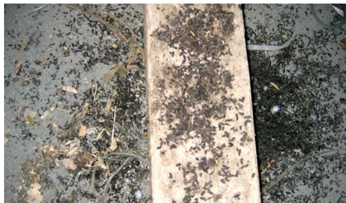
Fig. 9 The detailed view on the contaminants (droppings, hairs, gnawed material) fall down from the ceiling joists on the floor (photo: M. Fraňková)
